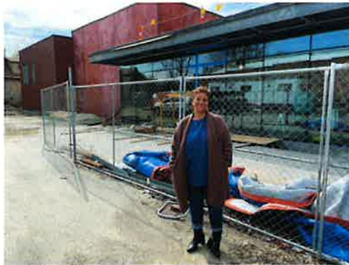
Brigitte McQueen, executive director of The Union for Contemporary Art at 24th and Lake Streets in Omaha, stands near the site of the Shirley Tyree Theater, which is under construction just south of the arts center.
