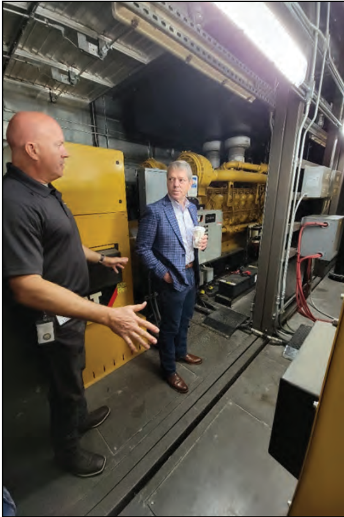
Building Division Administrator, Brent Flachsbart, explains the operation, testing, and maintenance process for the backup generator to Governor Pillen.
